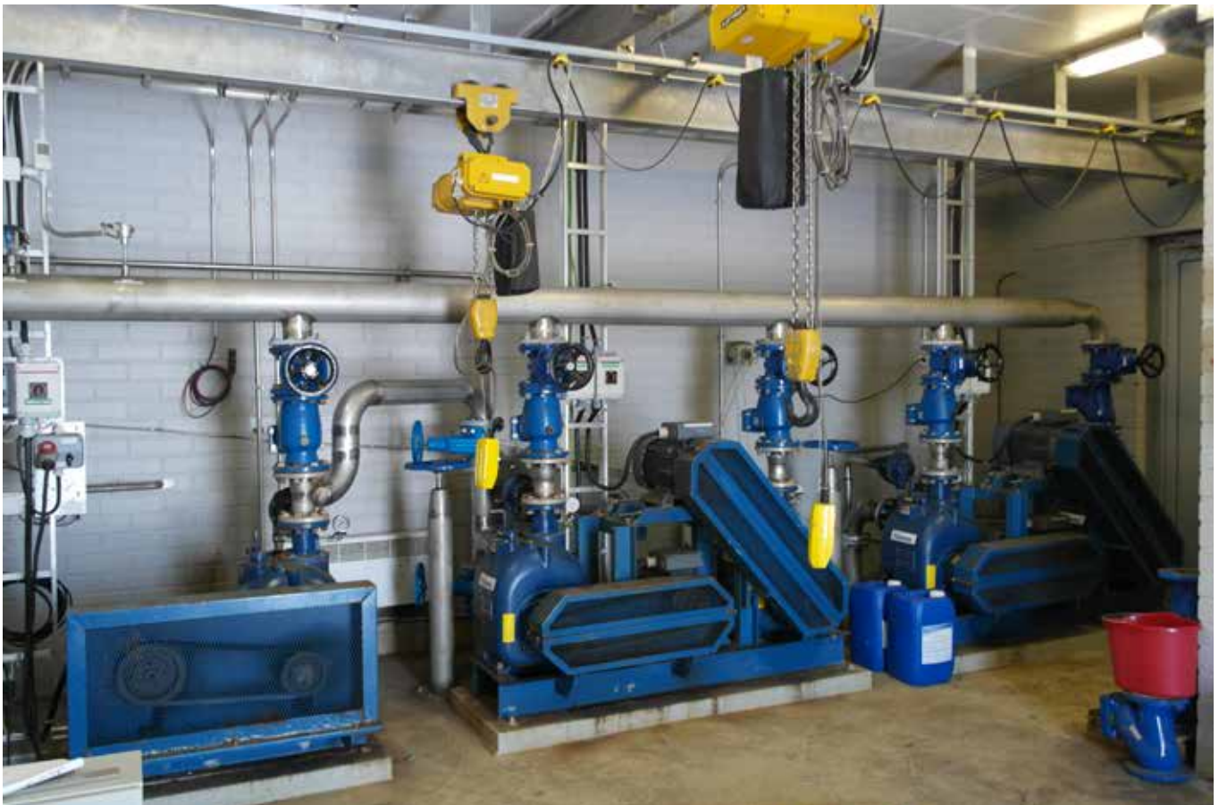
Pump station with in-built Malibu™ monitoring and automation system which ensures even flow of wastewater.
